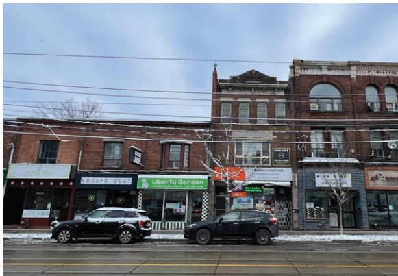
Brick masonry on the historic main street commercial buildings, located directly north of the Site (ERA, March 11, 2023).
