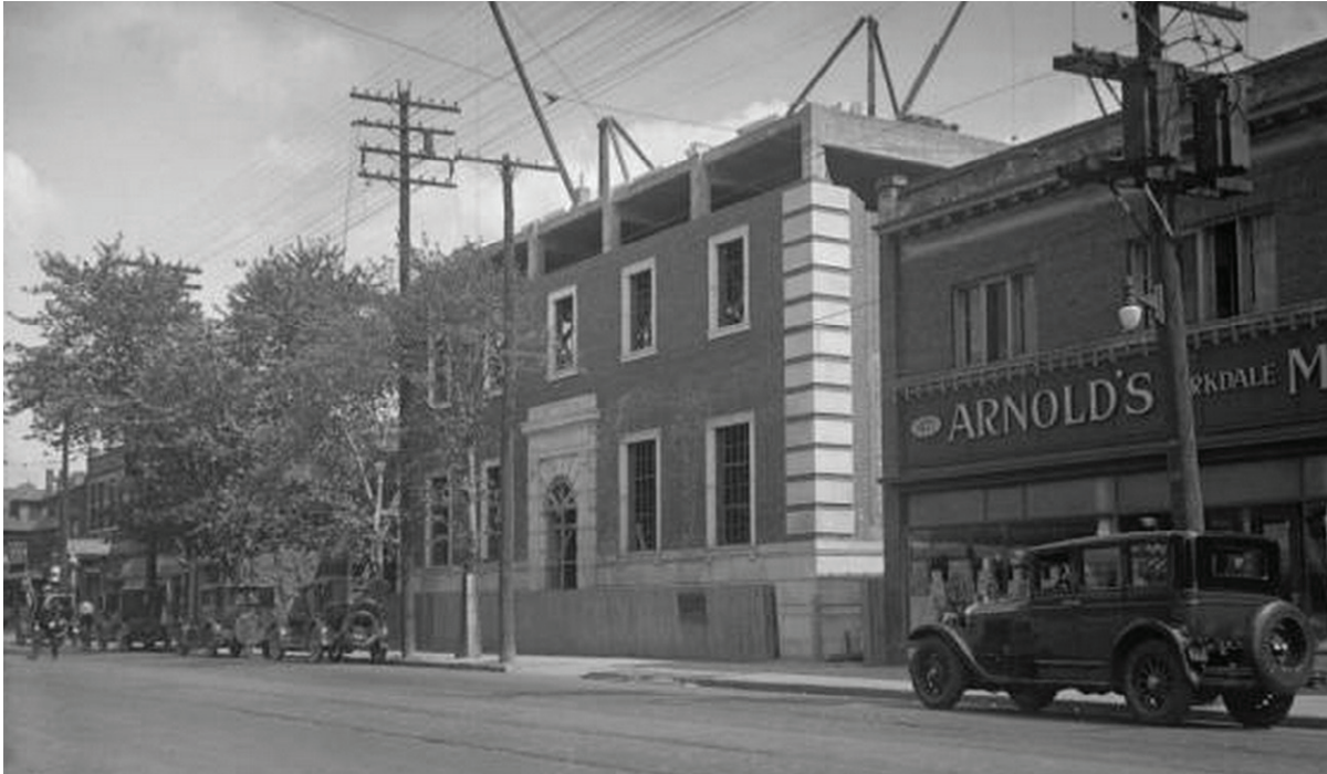
1927 photograph. Looking southeast on Queen Street West 1457 Queen Street West (Parkdale Substation) under construction (City of Toronto Archives).
