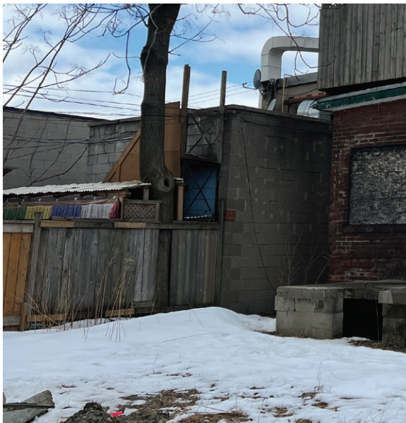
1439 Queen Street West: rear (south) and east elevations, as viewed from the parking lot at 1435 Queen Street West (ERA, March 2, 2023).
